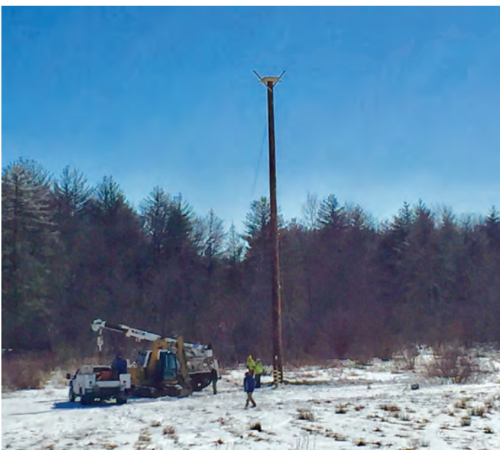
The platform and pole are finally up! Photo by Sue Bickford, Dover, NH, 2-26-19.
